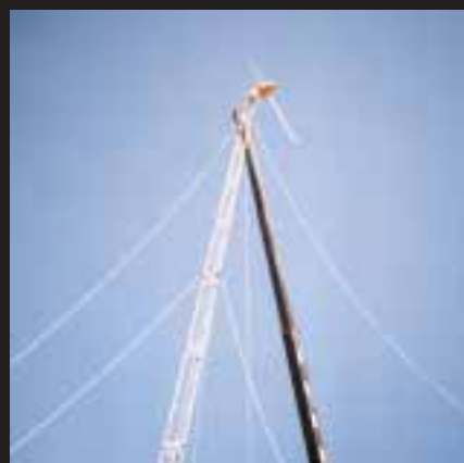
Snagged on the crane.
