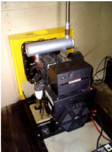
This large 7.5 kWatt diesel backup generator will last several lifetimes and be economical to operate as well.
