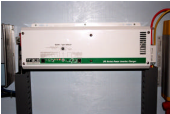
The modern off-grid world runs its electrical appliances on alternating current supplied by inverters such as this.
