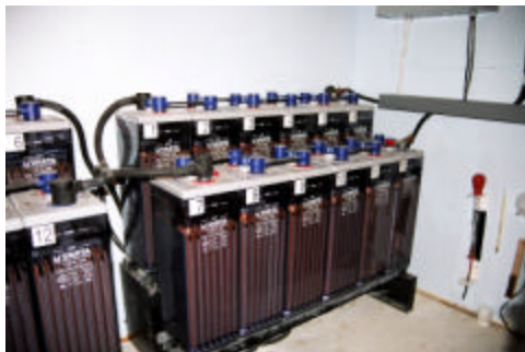
An off-grid system requires a means of storing the electrical energy generated by the renewable sources for later consumption. A sizeable battery bank provides the needed storage.
